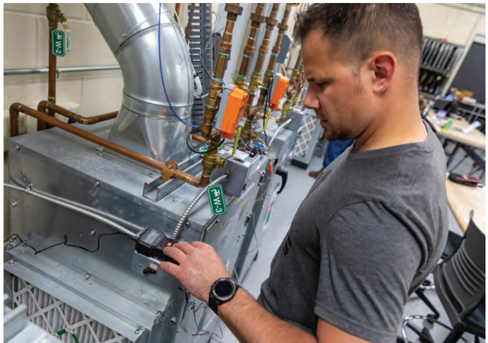
ACABT teaches students a wide array of skills, including how to check control signals to verify a motor's operating speed.
