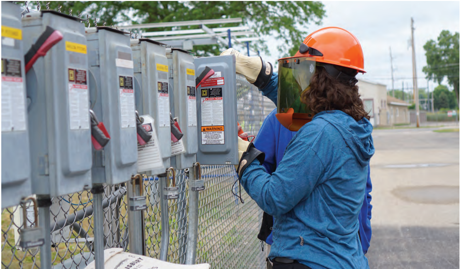
A student measures the electric potential across a solar photovoltaic disconnect switch, a maintenance task taught in CREATE's curriculum.
